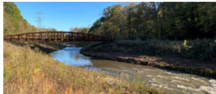
Example of a prefabricated bridge (112-foot span) across larger stream. This bridge came in two pieces and was set by crane.
