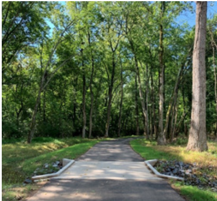
Greenway trail with shoulder, and small slab-top bridge/culvert to allow water to flow across floodplain without flowing over the trail surface
